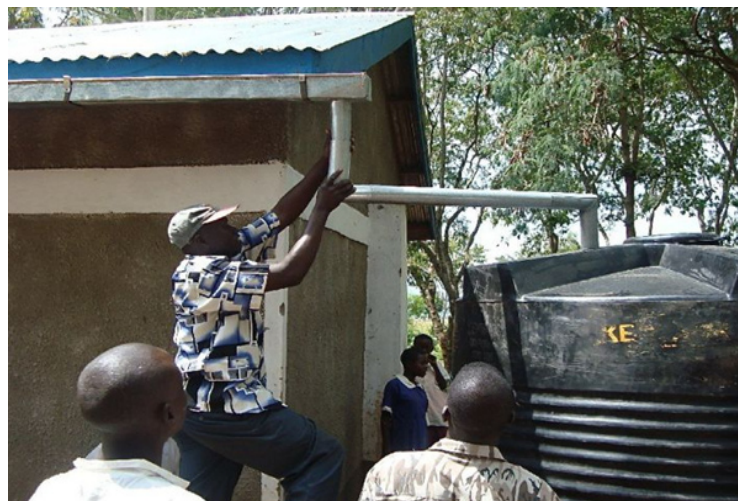
Fig. 2: RWH System in a public school 16
